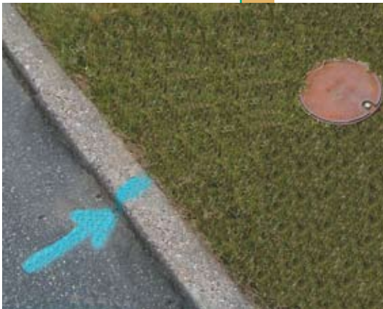
Water Meter Box
